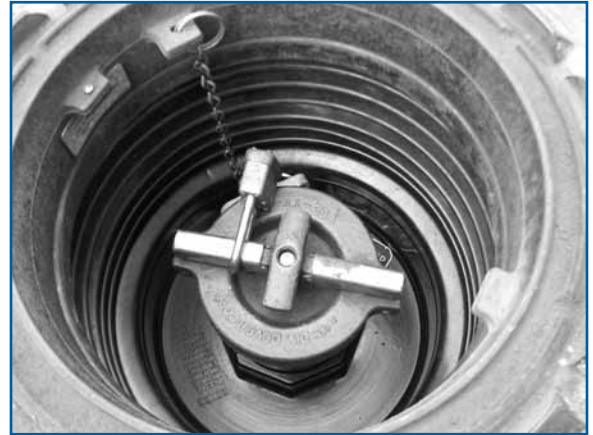
This spill bucket or fill well gets good marks for being dry and clean. See side article on the next page for ways to remove liquid from a fill well.
