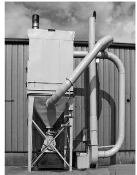
A baghouse in operation at a facility in Spokane
